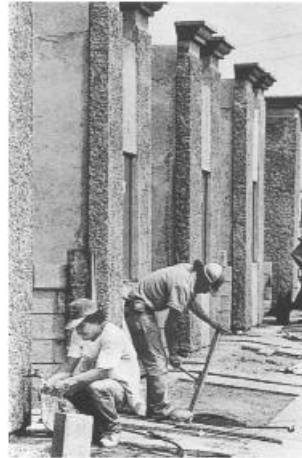
The Cooperative Housing Foundation is helping to provide homes for low-income families on the Mexico–United States border. Shown are construction workers at a nearly completed housing complex in Ciudad Juarez.
