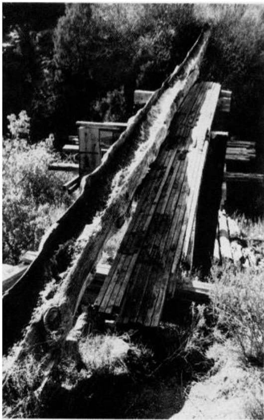
Hand-hewn wooden irrigation structures are used by Hispanic farmers in arid northern New Mexico to transfer water among their fields. Designwrights Collaborative of Santa Fe is helping the rural poor in the region protect their water rights.
