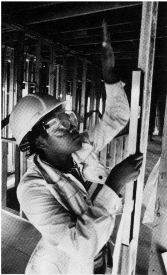
To prepare women for higher-paying jobs in the electronic and construction trades, the Foundation is supporting training programs in several U.S. cities. Here a trainee in Hartford, Connecticut, is learning on the job at a community-improvement work site.
