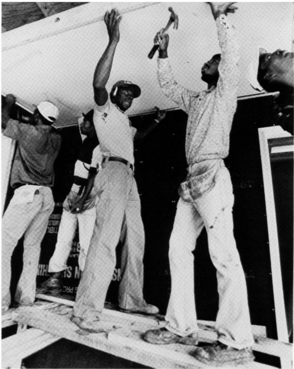
Teenagers work under supervision as construction aides in a housing program run by Mississippi Action for Community Education (MACE). A rural community development corporation supported by the Foundation since 1970, MACE offers poor Southern blacks such services as job counseling, literacy training, loans for business development, and help in forming credit unions and farmer cooperatives.
